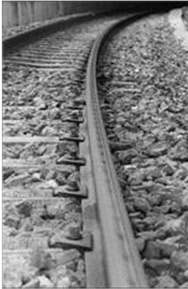
Fig. 6. Corrugations generated by normal operation.
