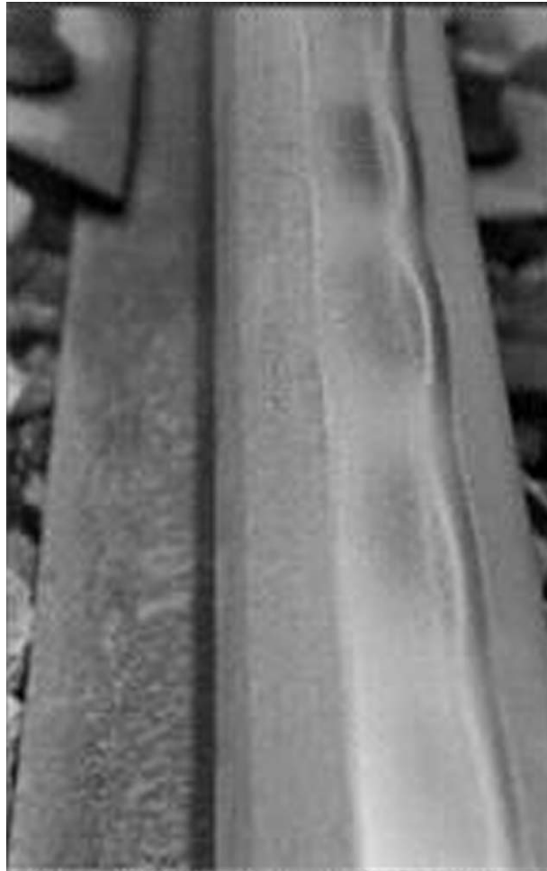
Fig. 7. Corrugations generated by normal operation.
